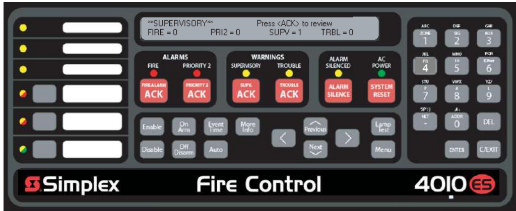
Figure 4-1. Interface Panel Showing Supervisory Condition
